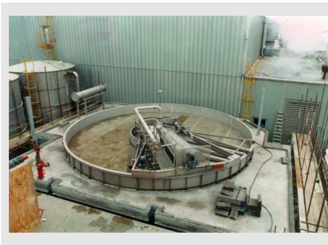
Example for a flotation plant (paper mill)
