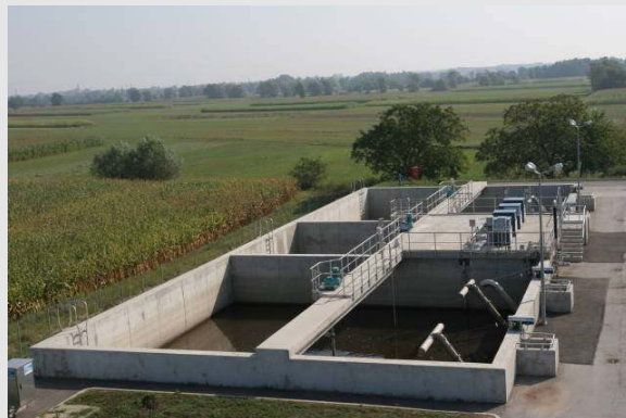
Wastewater Treatment Plant of the Croatian Town Virje (5,000 p.e.) operating with two SB-reactors, completely designed and equipped by Biogest International GmbH.
