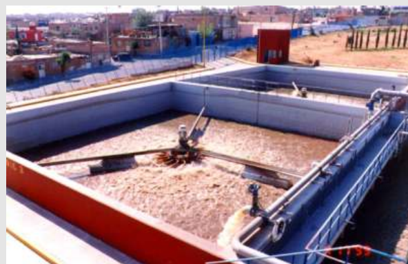
Since 1995 a wastewater treatment plant for a Mexican town (Aguascalientes) is operating based on the technology of Biogest International GmbH (floating surface aerators operating in totally five SB-reactors). The connection load is approx. 40,000 population equivalents.
