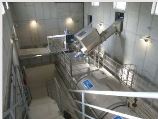
Pre-treatment station of the WWTP Koprivnica (max. hydraulic load = 1,600 m 3 /h).
