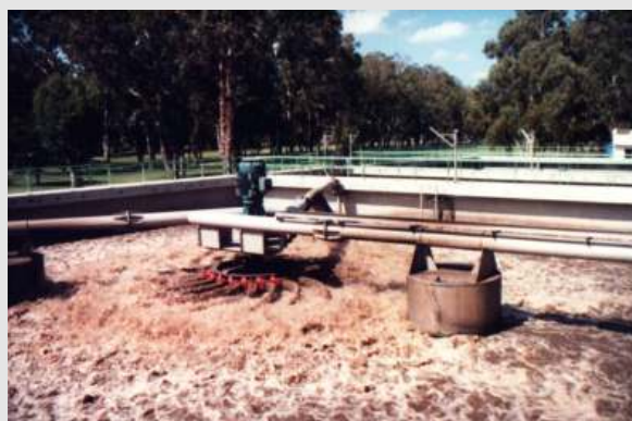
BSK®-surface aerator for a SBR-plant, operating in the Mexican town Celaya.
