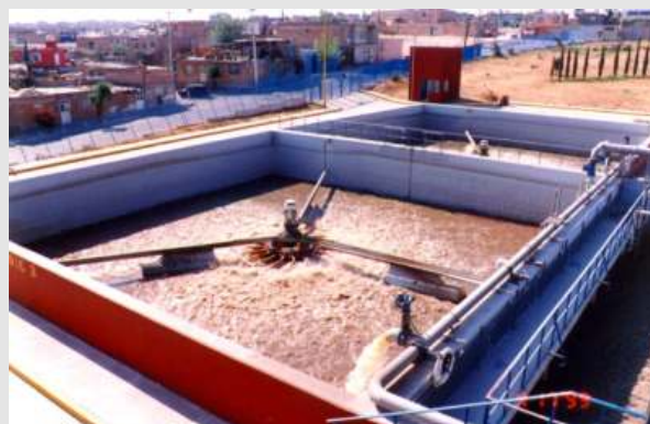
Since 1995 a wastewater treatment plant for a Mexican town (Aguascalientes) is operating based on the technology of Biogest International GmbH (floating surface aerators operating in totally five SB-reactors). The connection load is approx. 40,000 population equivalents.
