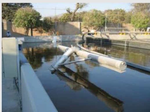
BSK®-clear water decanter installed at a WWTP in Mexico.
