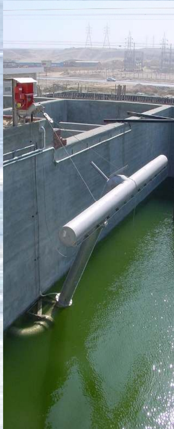
Clear water decanter DN 350 of the wastewater treatment plant Amreya (Egypt).
