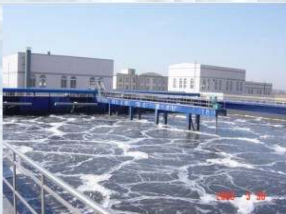
Picture no. 5: HyperClassic-Mixers for a big wastewater treatment plant. They are tasked to mix-up the activated sludge during the denitrification phase.
