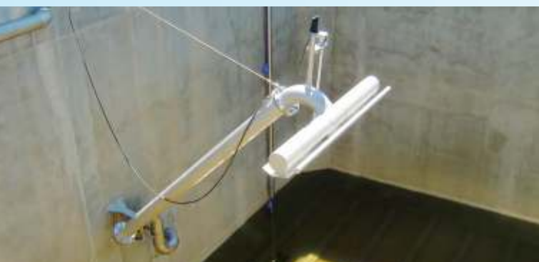
BSK®-Decanter of the WWTP Stepanovićevo (Serbia)
