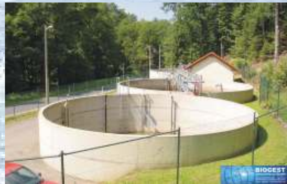
Photo no. 8: OTR-treatment system realised by use of two circular batch reactors. Connection load 3,000 p.e.
