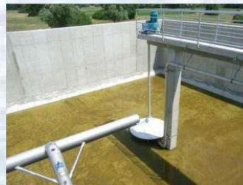
HyperClassic-aerator installed at a concrete bridge. In the foreground, a BSK®-decanter is positioned.
