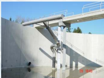
BSK®-decanter operating in a wastewater treatment plant next to Basel (Switzerland)
