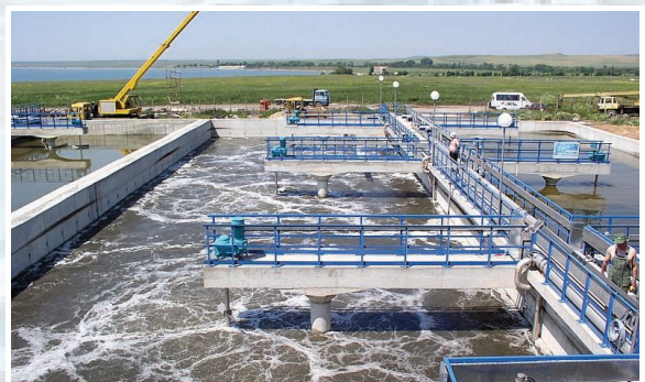
SB-reactor during aeration phase
