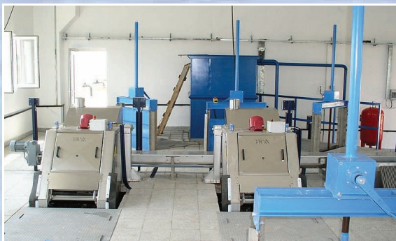
2-street screening system located in the operation building
