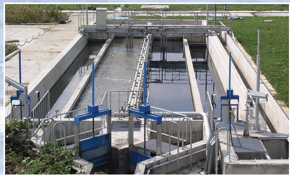
Inlet of the WWTP with valve and sand trap
