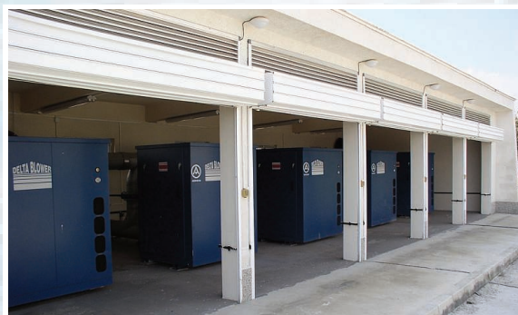
Station with 5 rotary blowers
