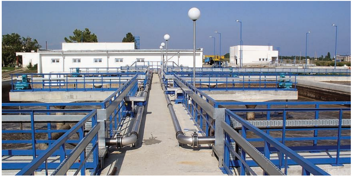
View from the service platform to the two SB-reactors
