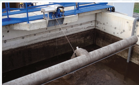
Clear water decanter with electrical winch
