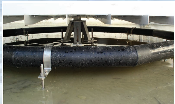
Detailed view of a mixing and aeration system
