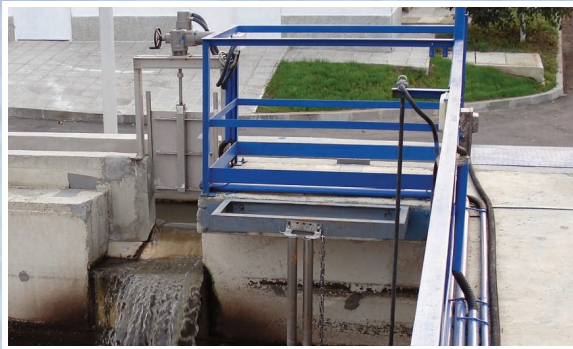
Automatically controlled inlet valve for reactor no. 2
