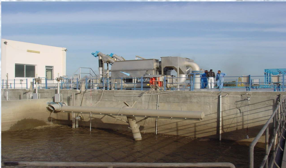
View from the turbine-platform to the pre-treatment station and BSK ® -Decanter
