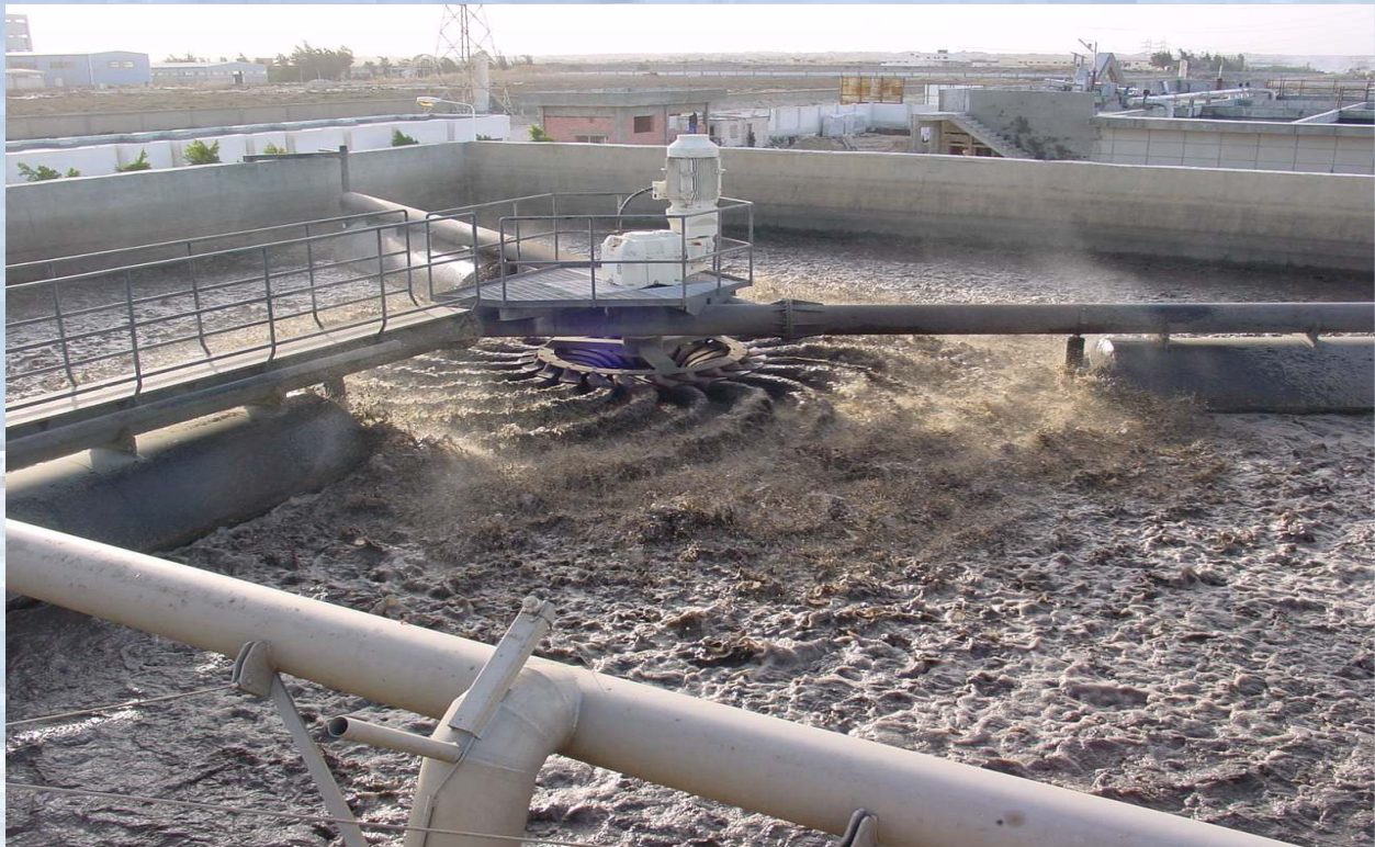
Key equipment of the wastewater treatment plant are floating BSK®-Surface Aerators, which guarantees perfect oxygen input capacity and proper mixing at low operation costs
