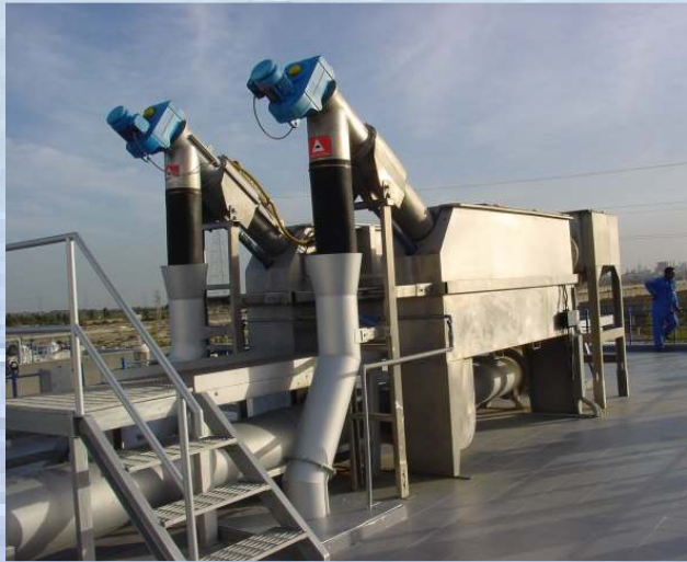
2-street automatic fine screen for mechanical pre-treatment
