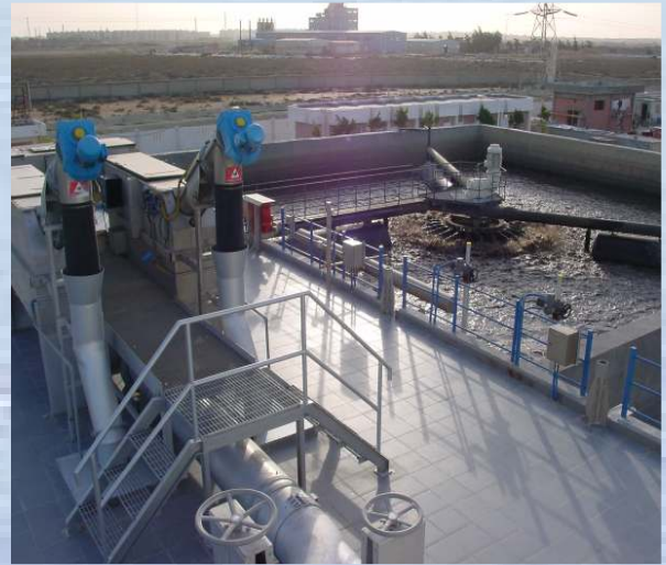
View from the operation building to the automatic fine screens and one of the SB-reactors
