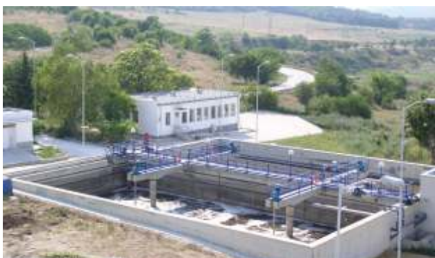
Installation SBR Commune Beloslav, Bulgarie
