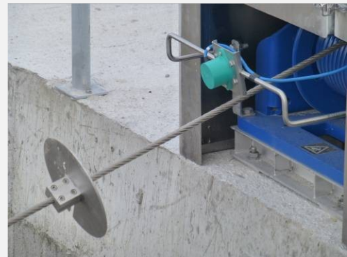
Emergency limit switch to prevent uncontrolled lifting of the decanter
