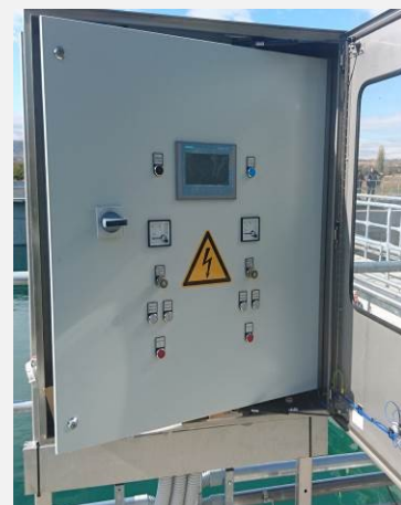
Example of a local stand-alone control system (plug and play), operating two (2) BSK®-decanters completely independent to the customer's PLC. This cabinet is equipped with a moveable cover with glass window. glass-window (for protection of dust).
