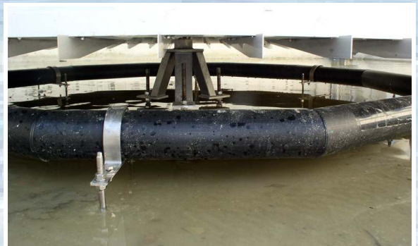
Detailed view of a mixing and aeration system
