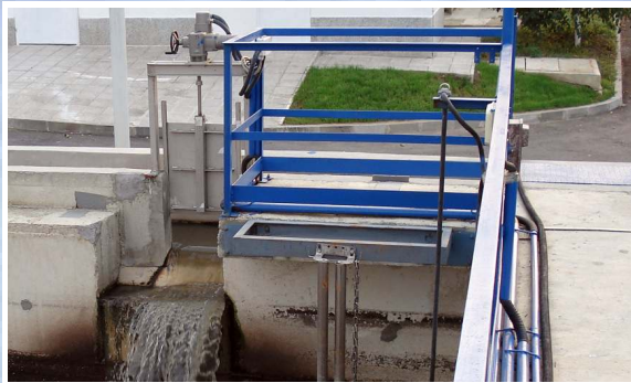
Automatically controlled inlet valve for reactor no. 2
