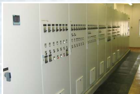
The control of the plant is performed automatically.
