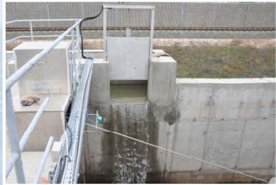
After pre-treatment, the wastewater is discharged by free flow and an inlet channel into the three SB-reactors
