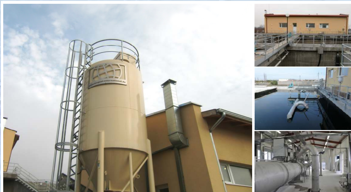
Biological wastewater treatment plant for the Bulgarian town Svilengrad
