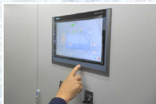
Next to the SCADA-system all data can be read by a state-of-the-art touch panel.
