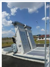
automatic coarse screens for first mechanical pre-treatment
