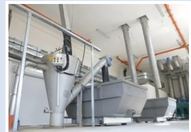
collecting of solids and washed sand for final disposal
