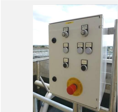
Example of a local switchbox for one BSK®-decanter. The cabinet could be produced by use of glass fiber reinforced plastic (GRP) or stainless steel. Moreover, the front side could be covered by a moveable door with glass-window (for protection of dust).
